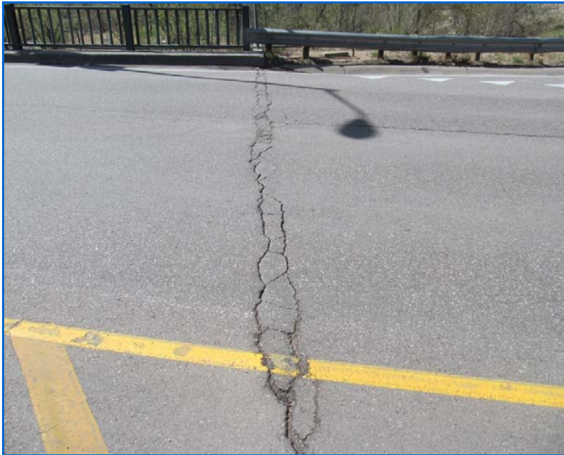
CSG-F.85-08.23 Transverse cracking with impending potholes in asphalt at west.JPG
