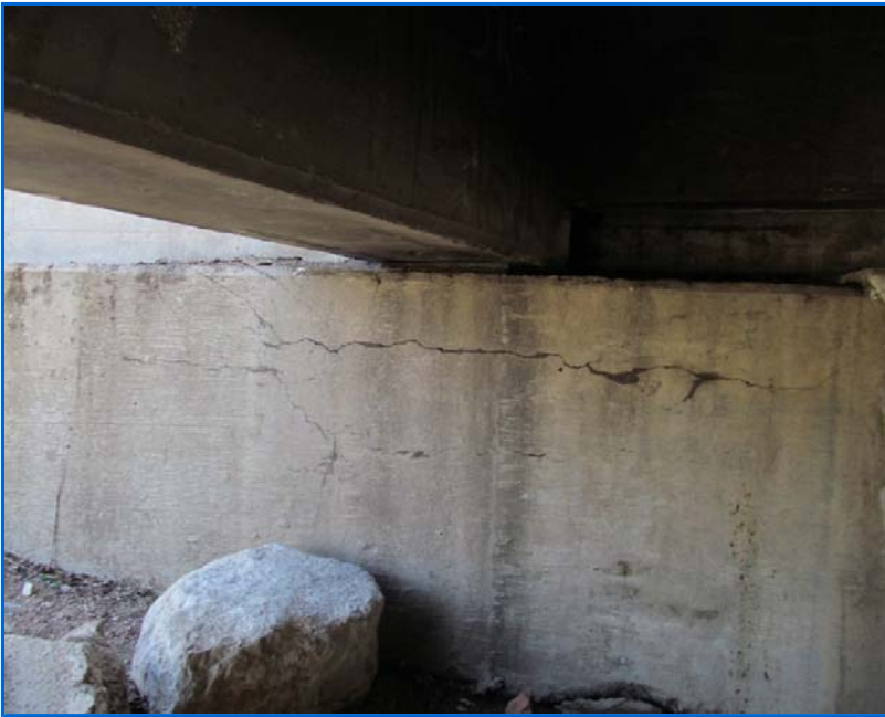
CSG-F.85-08.23 Horizontal cracks in abutment at A5.JPG
