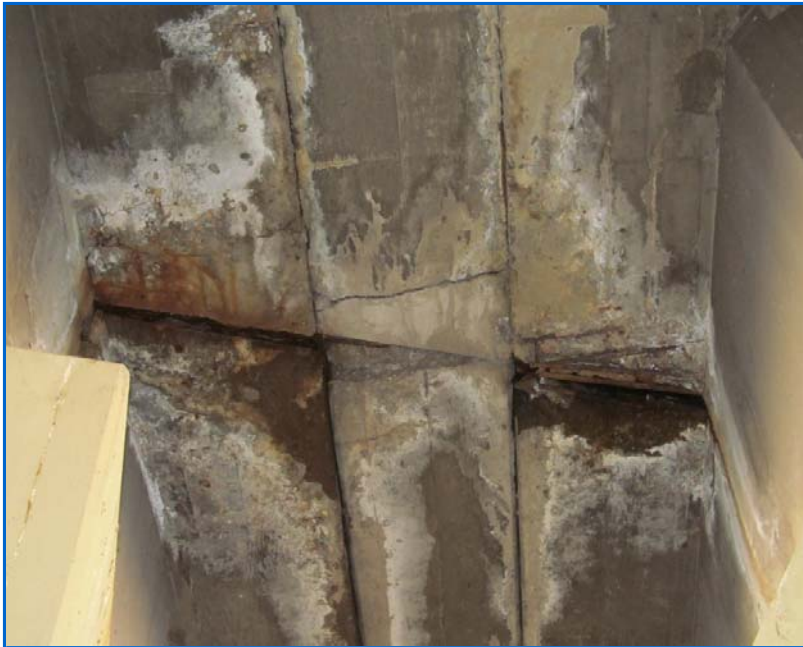
CSG-F.85-08.23 Cracking, spalling, exposed rebar, and active leakage below median at P2.JPG
