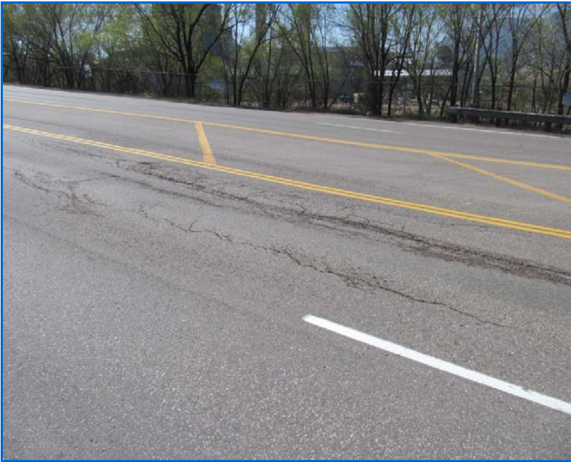
CSG-F.85-08.23 Ruts in westbound travel lane.JPG
