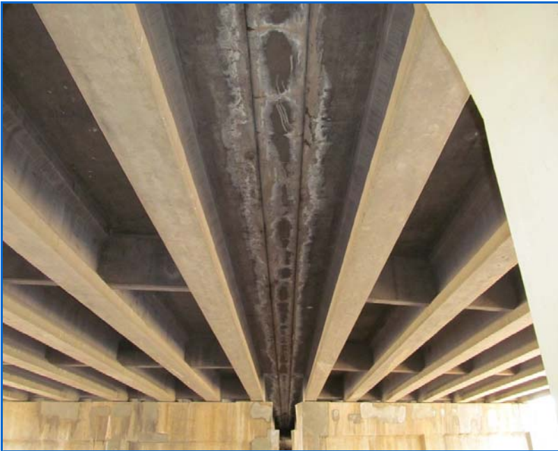
CSG-F.85-08.23 Chloride staining and efflorescence full length of median.JPG
