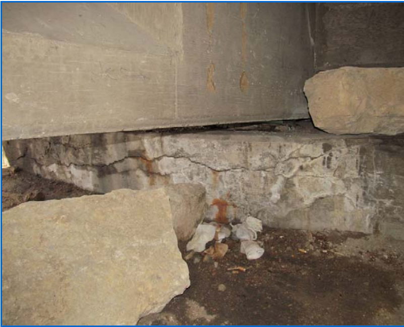
CSG-F.85-08.23 Cracking and delamination with efflorescence and rust staining at A1 at southwest.JPG
