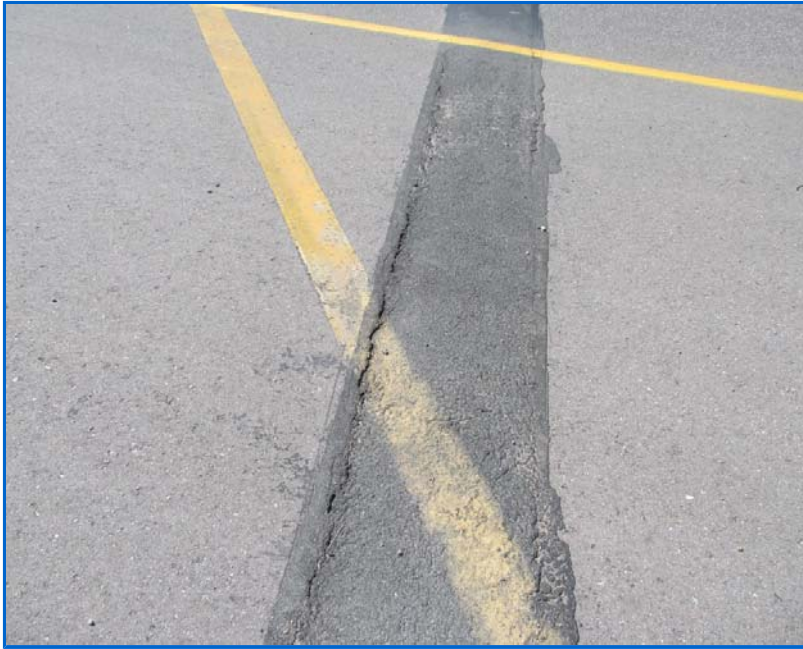
CSG-F.85-08.23 Typical debonding failure in plug joint.JPG
