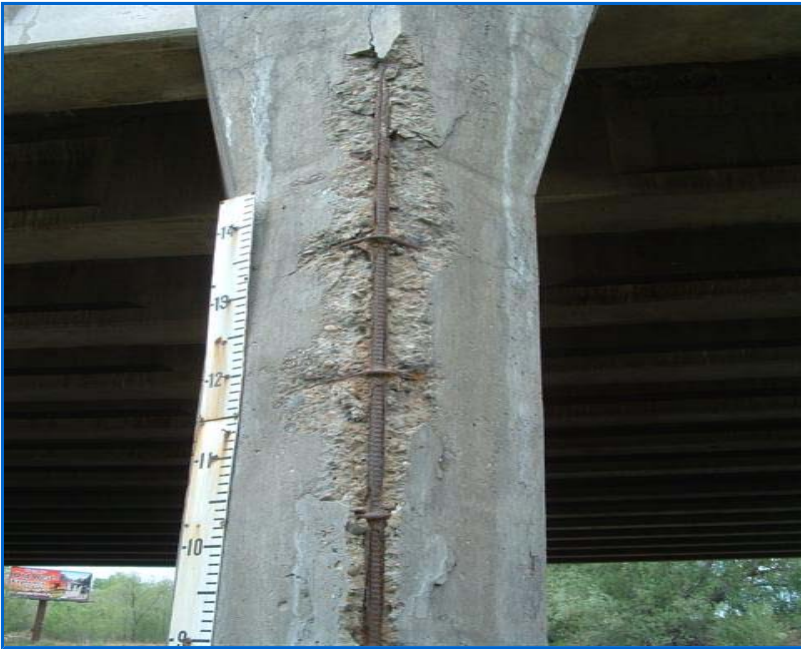
CSG-F.85-08.23 SPALLING WITH EXPOSED REBAR IN SOUTH END (2).JPG
