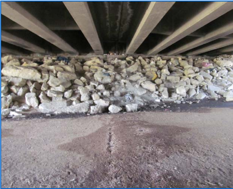
CSG-F.85-08.23 Active leaking underneath bridge at median.JPG
