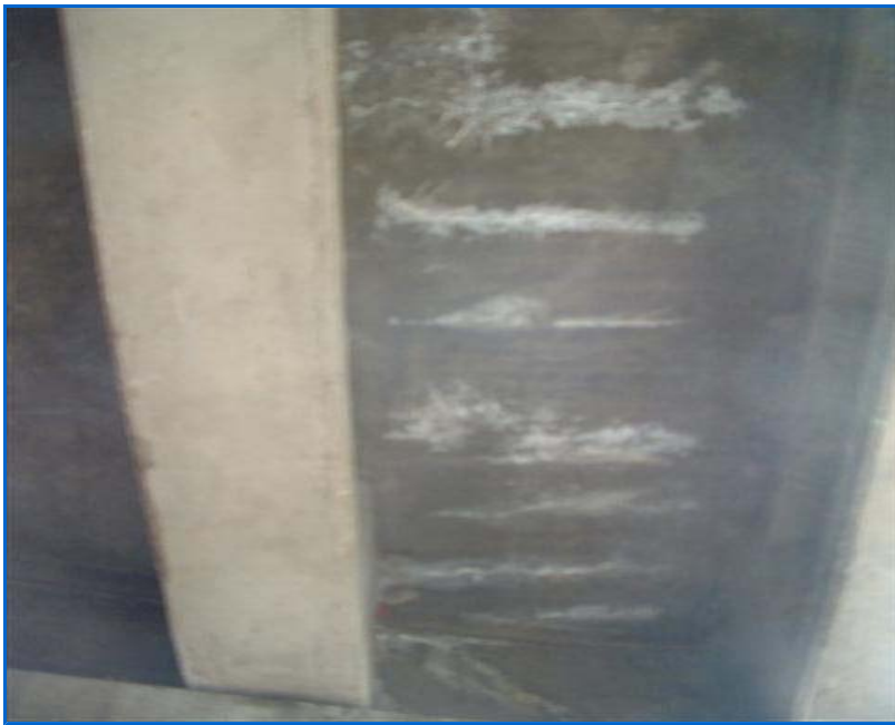
CSG-F.85-08.23 CRACKS WITH EFFLORESCENCE IN SOFFIT.JPG
