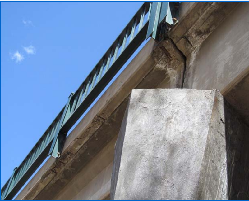
CSG-F.85-08.23 Spalling with exposed corroded rebar at south edge of deck at P4.JPG
